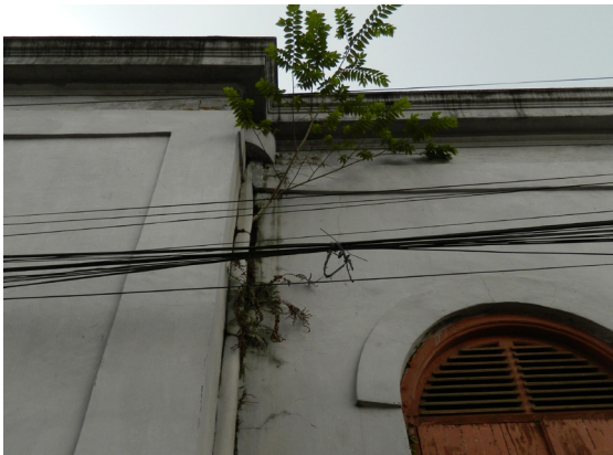
Gutter and Biological Growth
