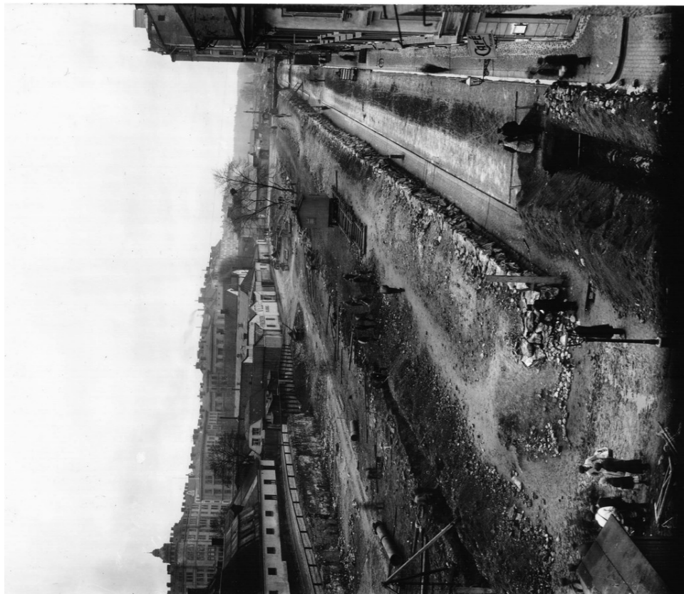
Sprängstensmur in the middle of the photo - traditional for the Swedish context Available at: https://www.bjornpatricks.com/BP2/Sveavaegen/Sveavaegen.html
