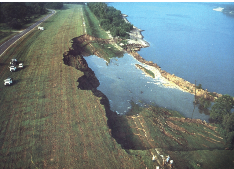
Figure 2.2: A levee failure in Ascension Parish, Louisiana, from Rogers (2016)
