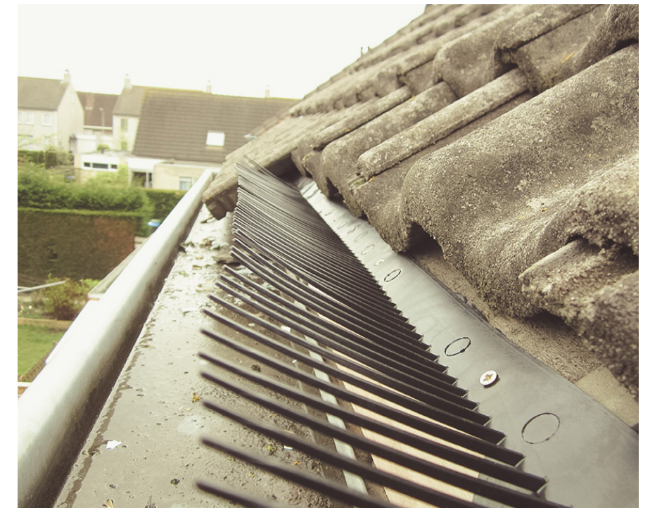
Animals should not come too close. Bird scraps keep birds out under roof tiles. (Adapted from Traas Building Care, n.d.)
