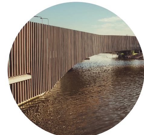
Bat bridge (Rutting, 2015)
