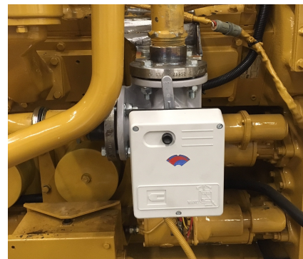
Figure A.10: Cooling three-way valve placed with electric motor
