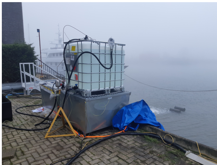
Figure A.5: Dip tray with Methanol IBC container used as fuel tank
