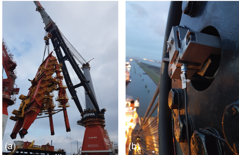
Figure C.1: Pictures of “Aegir” measurement, showing; (a) second lifting operation, and (b) sensor installed on shaft.
