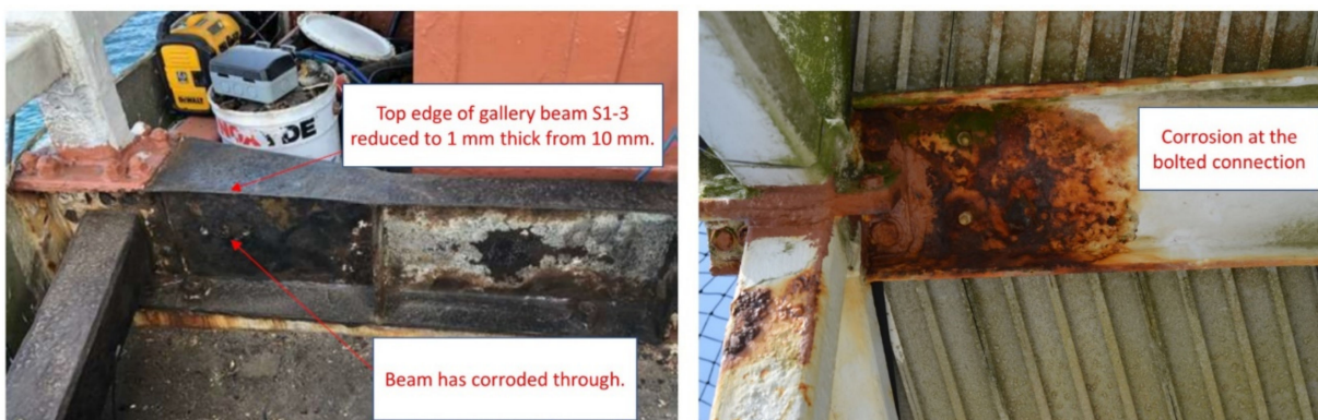
Figure 4. Examples of corroded areas of the helideck [courtesy of Trinity House].
