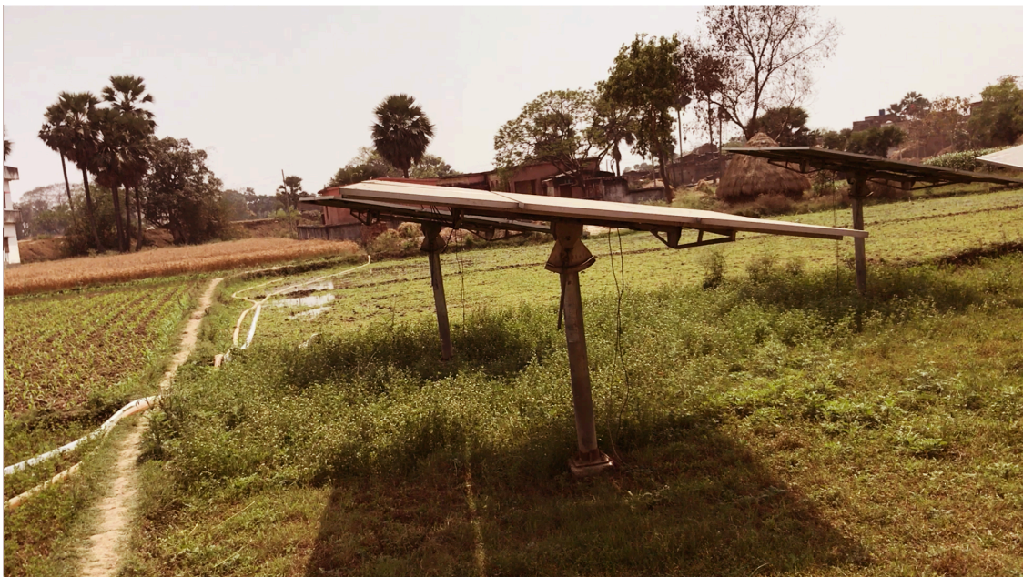
Figure 7.11: Three of the six solar panels used power to the pump that irrigates the land, but powering nothing else
