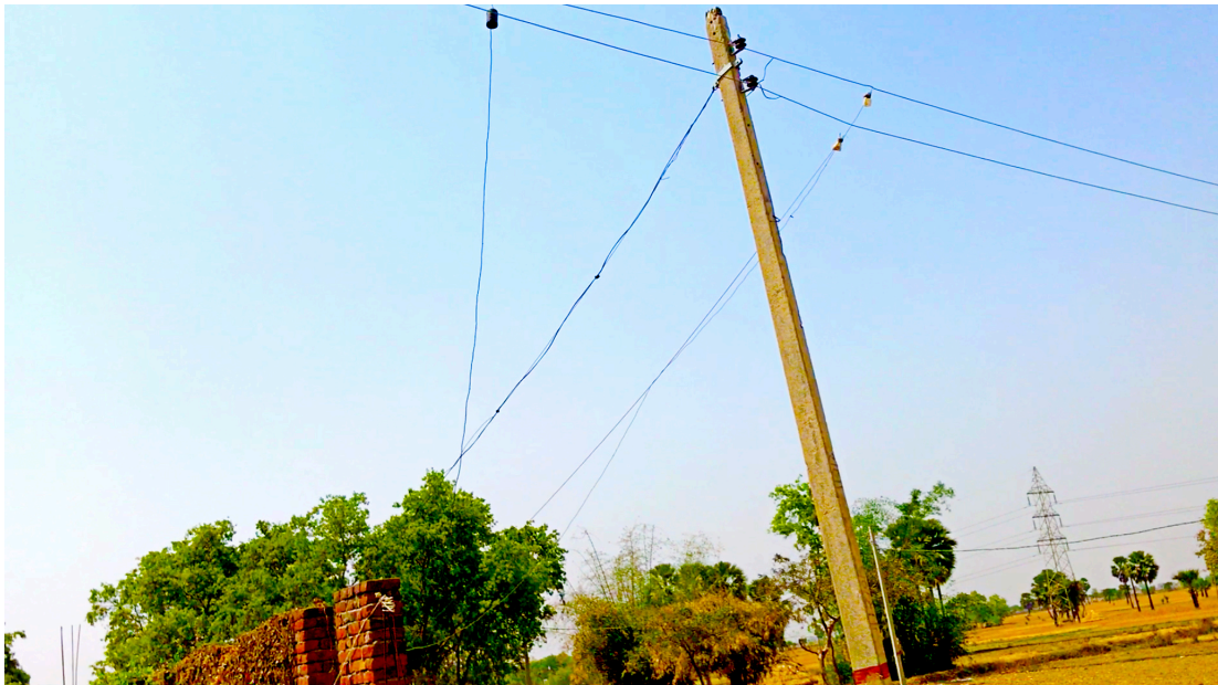
Figure 7.8: Illegal connections to the central government grid
