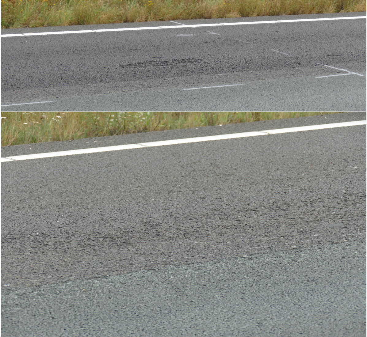
Figure 5.3: Illustration of ravelling on the road sections between driver location signs 203.3-203.5 on the carriageway 1HRR of the A50.
