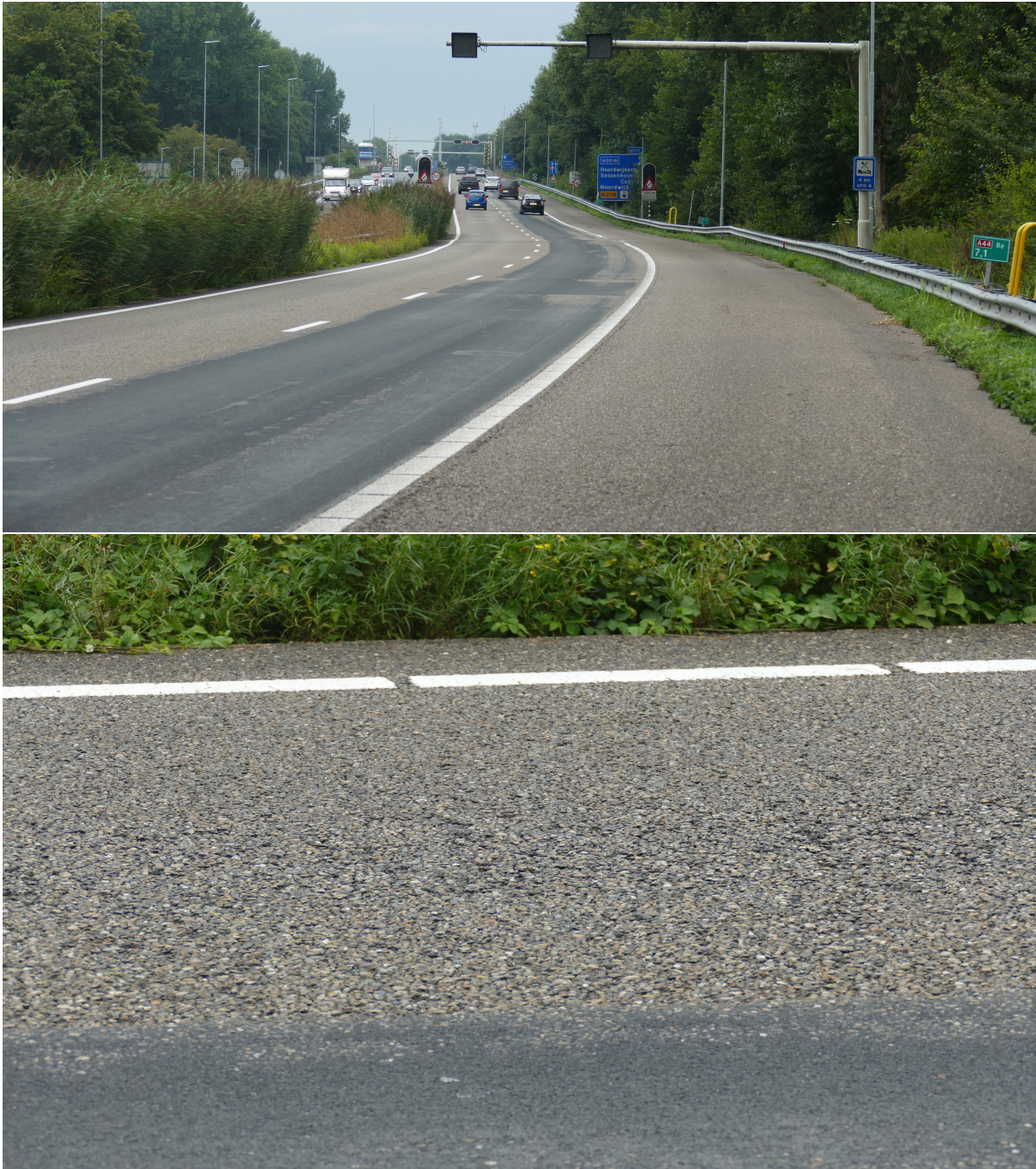
Figure 5.2: Illustration of (ravelling on) the road section starting at hectometer post 7.1 on the carriageway 1HRR of the A44.
