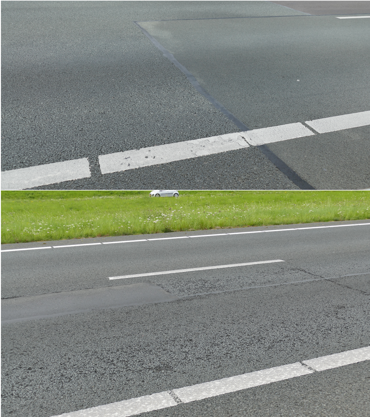
Figure 5.4: Illustration of transition in ravelling between two different surfaces and severe ravelling on the road sections starting respectively at hectometer post 282.7 and 287.3 on the carriageway 1HRR of the A6.
