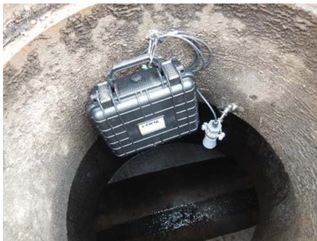
Figure 11.23 LoRaWAN prototype including water level sensor (MaxBotix) installed in a sewer manhole. Source: Eawag.
