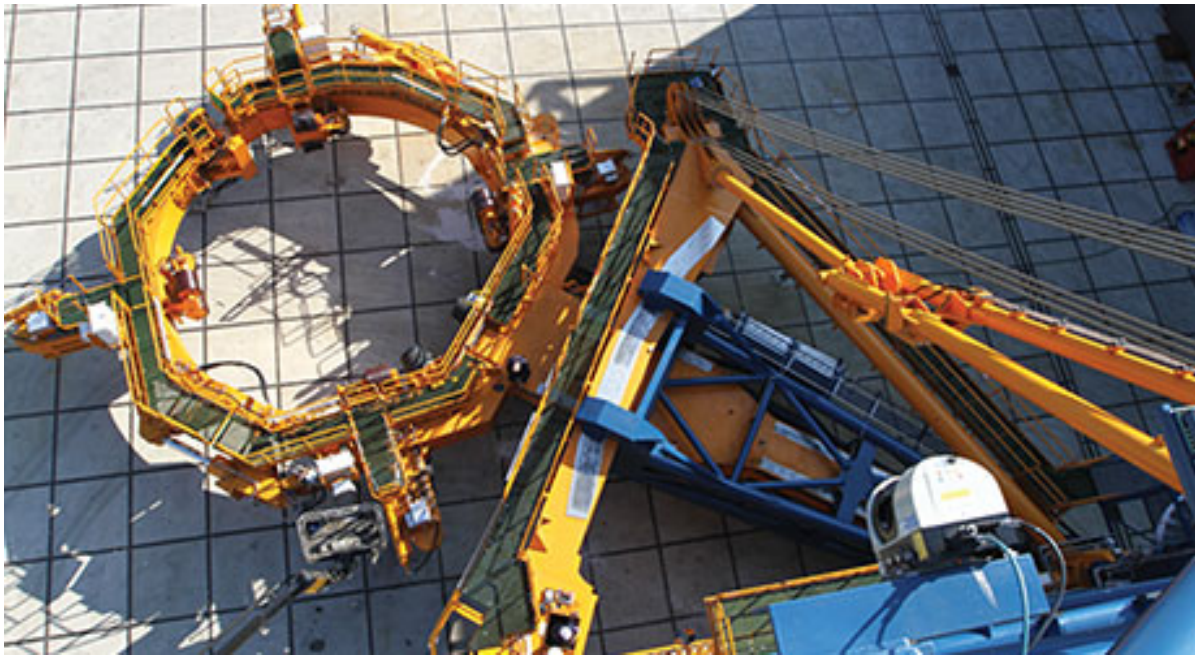
Figure 2.7: An example of a gripper frame holding the monopile upright during the hammering phase of the monopile installation [33]. This gripper frame has been used on van Oord's jack-up vessel Aeolus.
