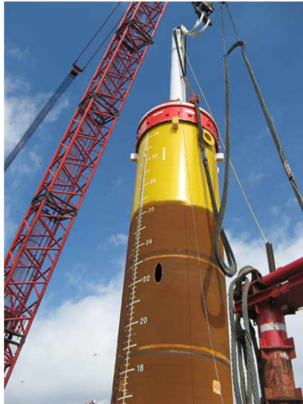
Figure 2.4: An example of an monopile and hydraulic hammer at the top. The monopiles are hit with the hammer and driven into the seabed. 2
