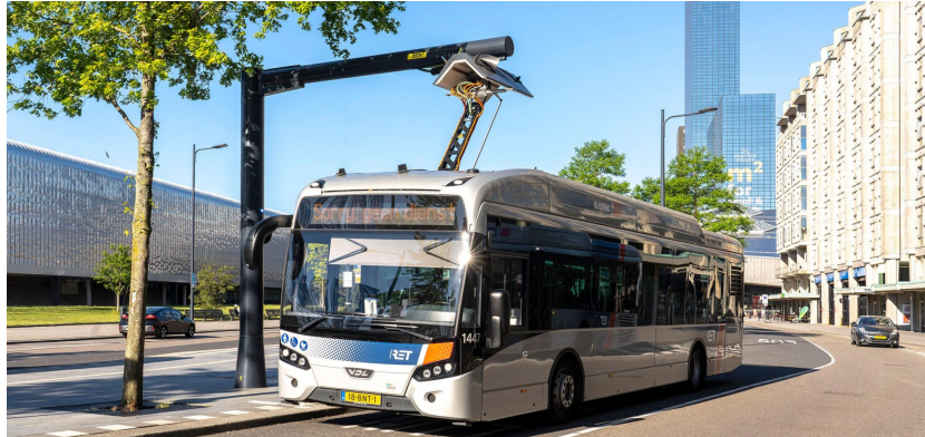
Figure 4.6: An RET pantograph charger at the central station of Rotterdam
