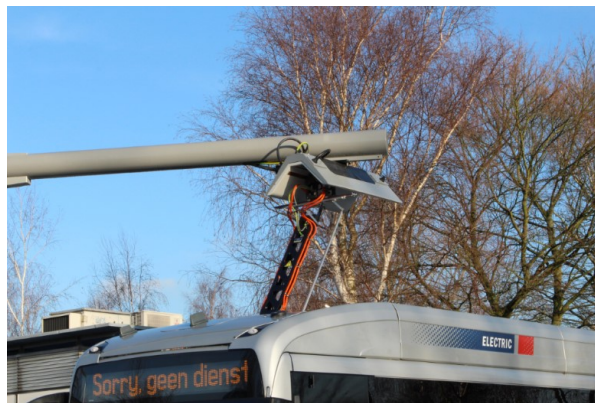
Figure 4.7: A pantograph charger of the RET in Rotterdam
