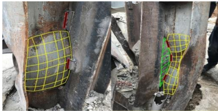
Figure 5. Buckling deformation and welding of C6 steel column. From the Investigation Report on the Collapse of Xinjia Hotel, Quanzhou City, Fujian Province.
