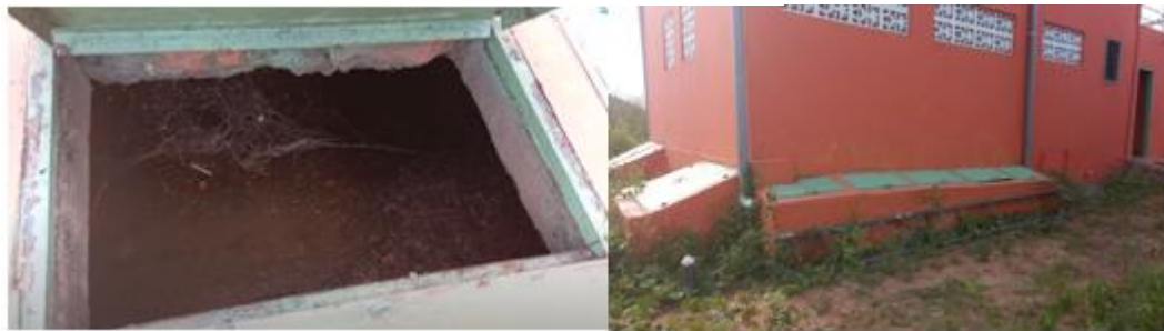
FIGURE 6: LEFT: OPENED SOLID LIQUID SEPARATOR. RIGHT: ACCESS TO THE SOLID LIQUID SEPARATOR FROM THE OUTSIDE.
