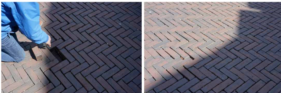
Figure 5 | Case #29 has been assigned the root cause Incomplete knowledge about the interactions of SUDS with other urban systems. Due to the impact of cars as well as street sweeping, the joints of the permeable pavement bricks vanished. This decreased the overall performance of the SUDS, i.e., the stability of the road surface.
