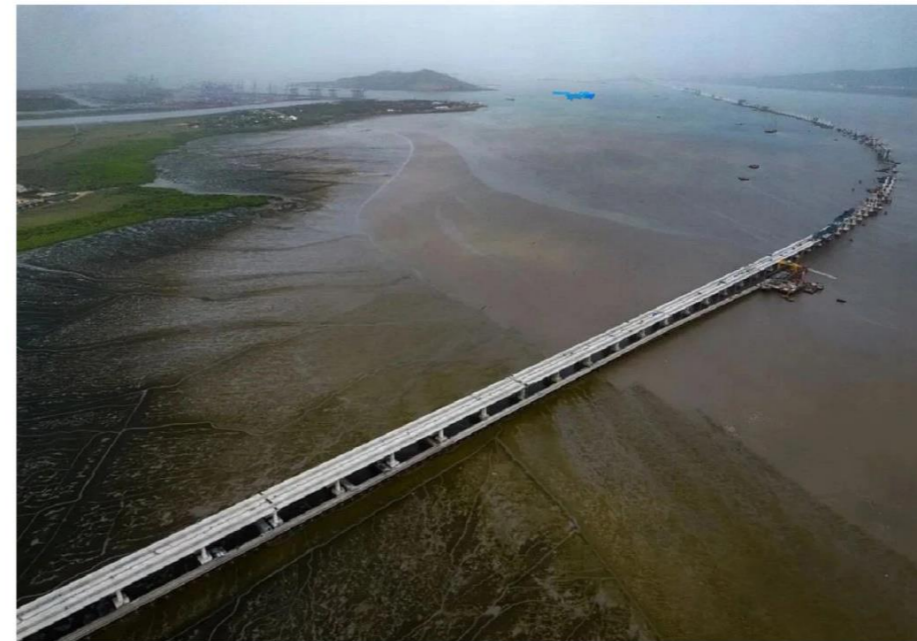
An actual visual of the bridge under construction captured in September, 2022. Showing its material impact on the landscape. Bridge due for completion in November 2023. Image Source : @cldbage/Twitter
