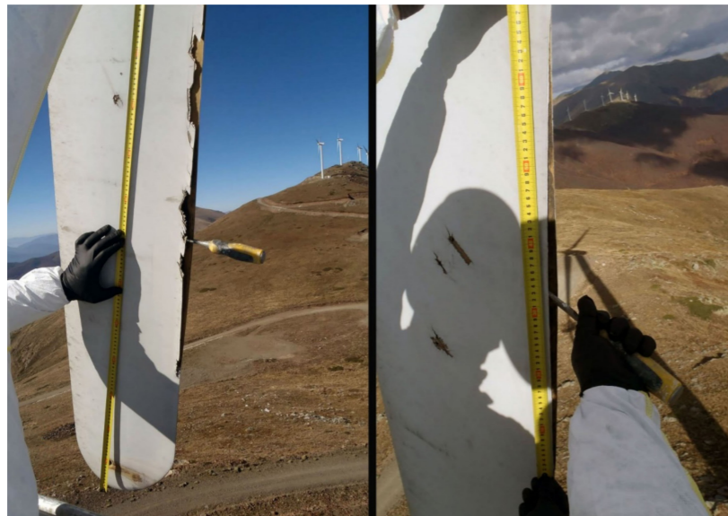
Figure 15: Shell debonding on join line between shell halves (Katsaprakakis et al., 2021).
