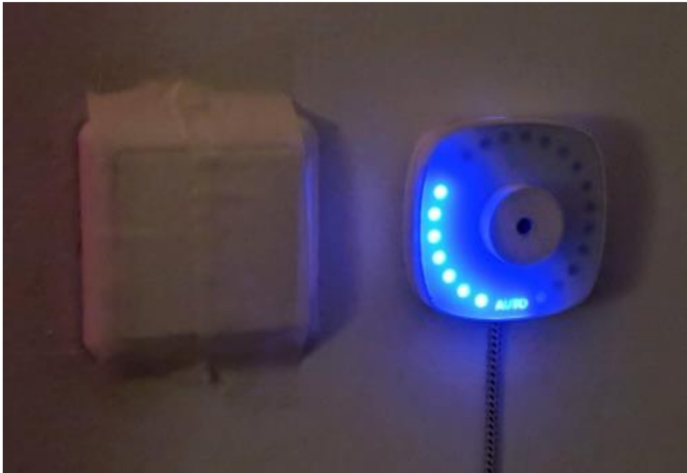
Figure 43: The dimmer next to the light switch while in automatic mode.
