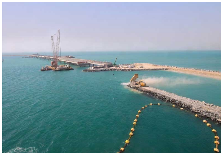
Figure 2.20: Expansion of the Jebel Ali Port. The construction is protected by a rubble mound breakwater to prevent erosion. (source: Logistics Middle East).
