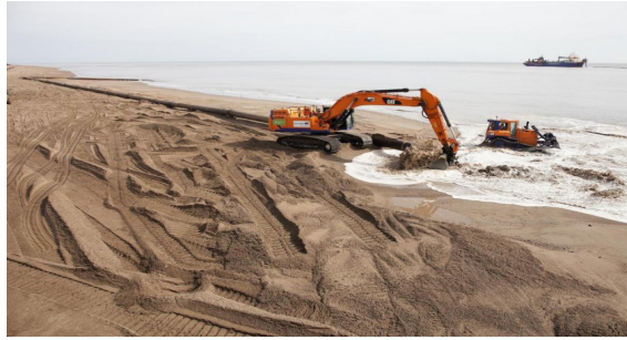
(c) Beach nourishment under construction along the coast of Lincolnshire, UK. (source: Van Oord).
