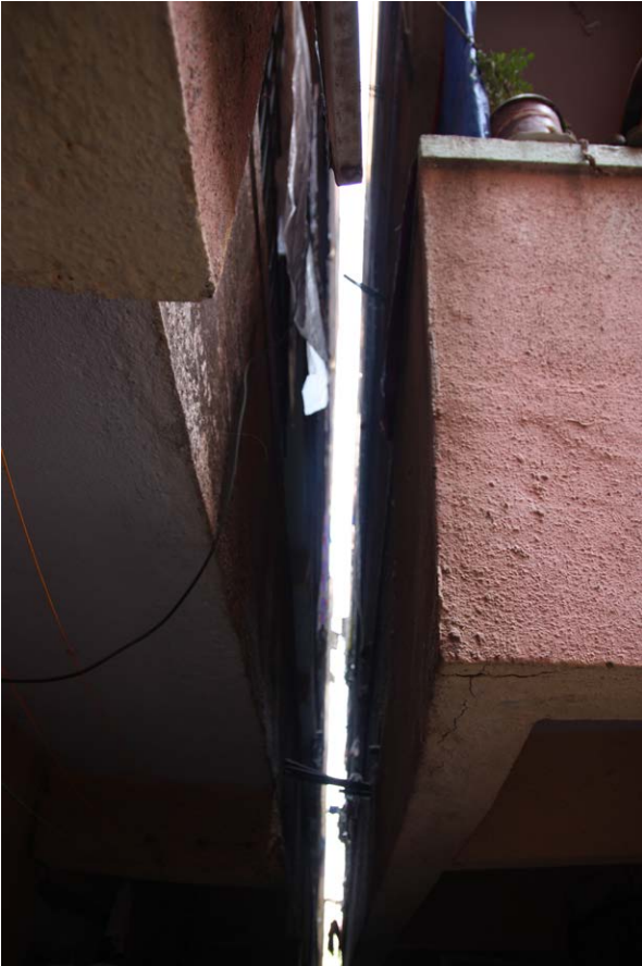
Lack of daylight
