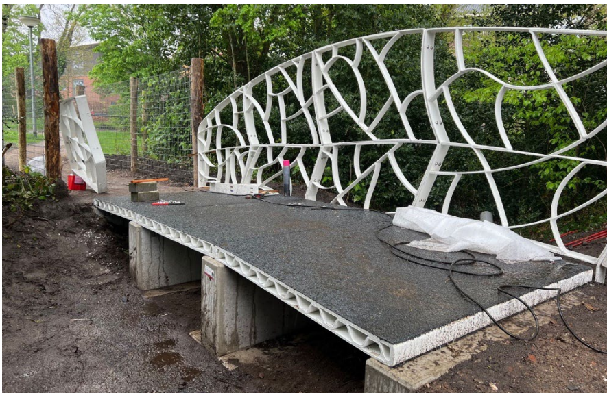
Figure 2-7 3D printed pedestrian bridge in Putten from Royal HaskoningDHV, Atelier Dutch, and Nedcam [14]
