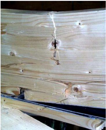
(a) Ductile beam failure [44]
