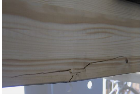
(b) Tension failure for beam in bending
