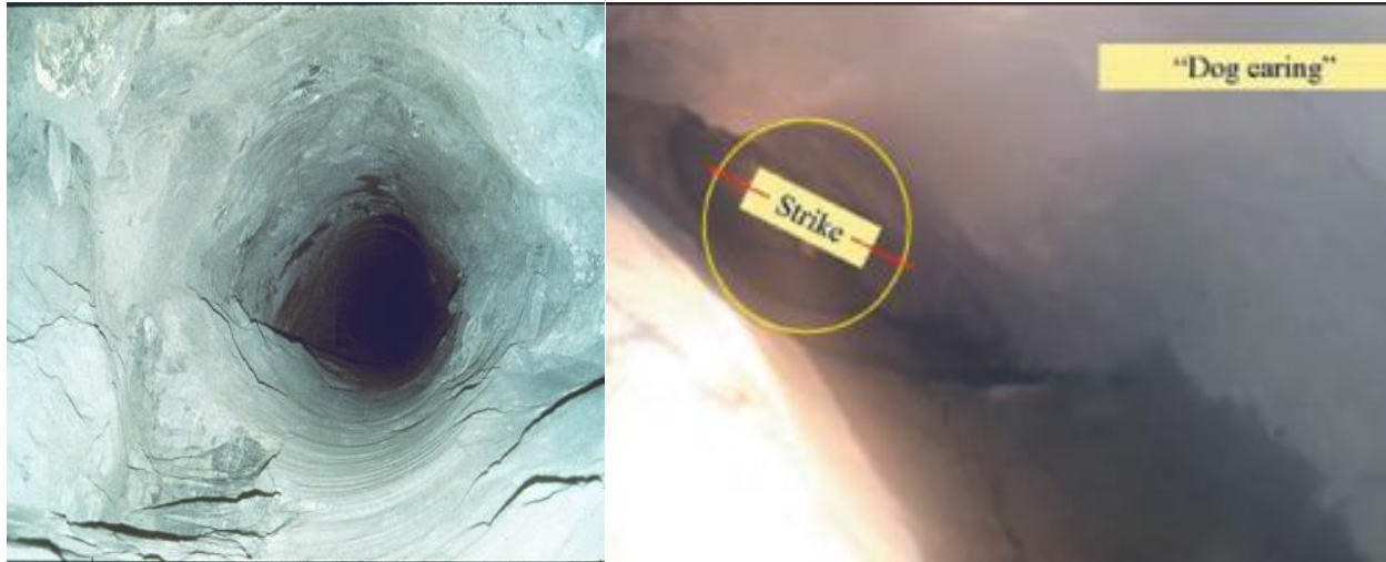
Figure 2 Dog earing occurs in high stress conditions (Hadjigeorgiou, Mercier-Langevin 2008b) and (Hart 2006)
