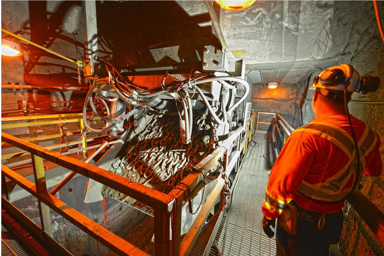
Figure 9 Chute loading station where truck is loaded below the steel frame. Chute is equipped with chains and water spray to smooth material flow and decrease dust emissions. (Variant Mining)
