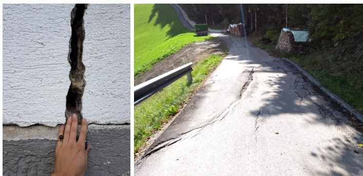
Figure 1.4: Damage to a house (left) and infrastructure (right) in Vögelsberg due to slope movement. (left: image courtesy of Thomas Zieher, right: image by the author, October 2018)
