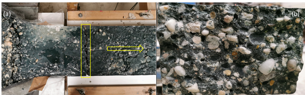
Fig. 11. Cracking (a) and the fracture surface (b) of the concrete.
