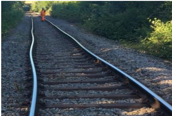
Figure 6.18 Rail deformation laterally (NetworkRail_news, 2019)
