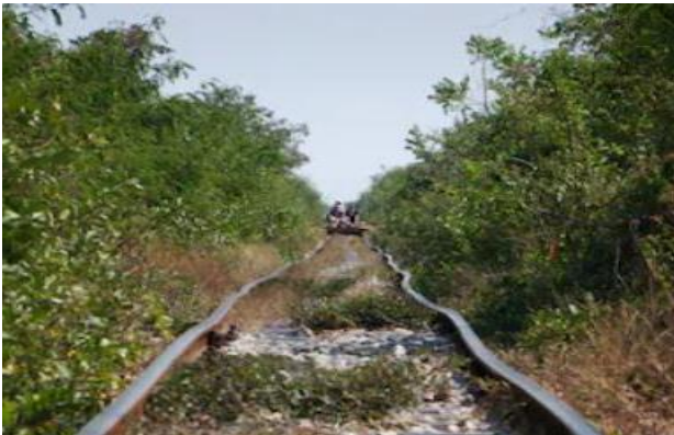
Figure 6.17 Rail deformation vertically (heat_distortion, 2009)
