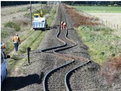
Figure 2.29 Rail Buckling (Railway Buckling, 2016)
