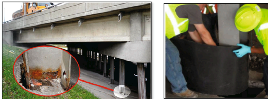
Fig. 15. One of the 49 corrosion damaged piles in I-70/I-270 Interchange (USA) that were repaired with wrapping FRP technique [98].
