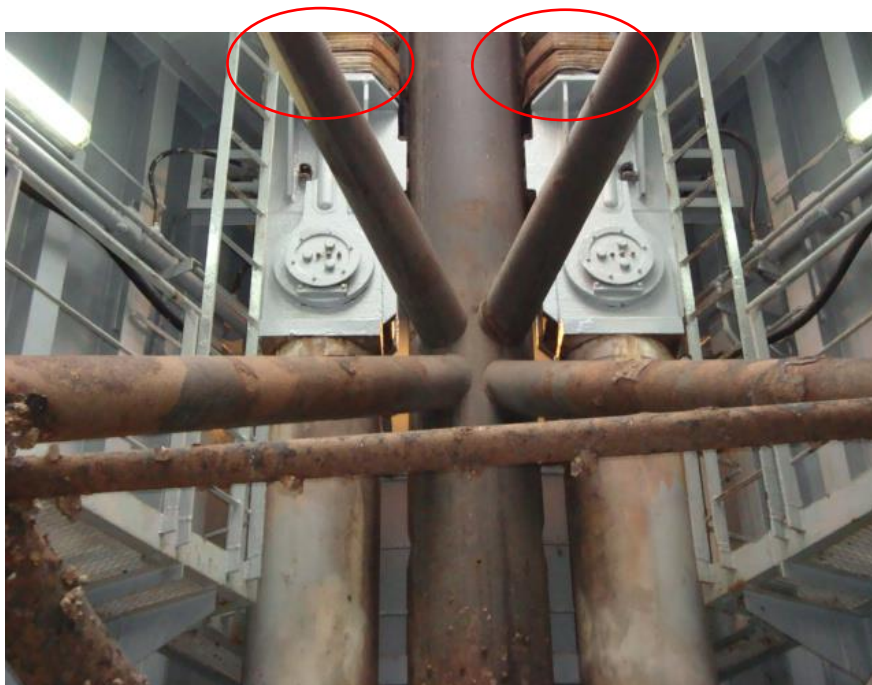
Figure 4-10 Holding pins inside the jack house
