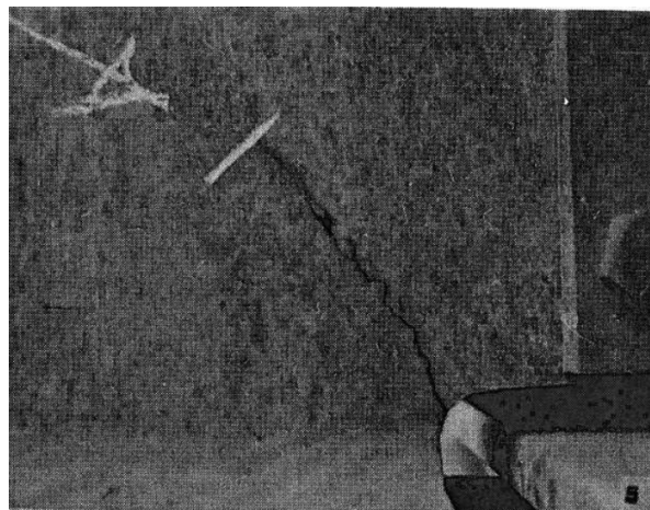
Figure 4.5: Path of the crack propagation [67].
