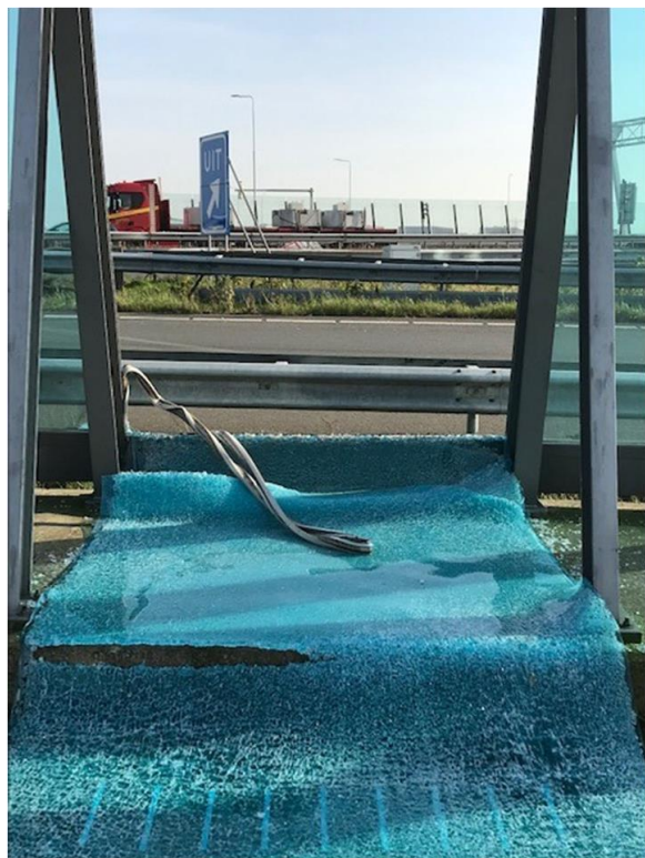
Fig. 1: Failed tempered laminated glass sound screen panel
