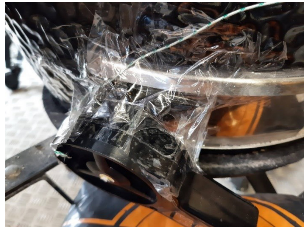
Figure 58. sealing the anemometer to the damper air inlet to measure displaced air.
