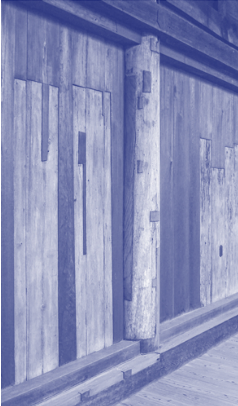
Fig 7: Ryūfuku-ji Temple as a patchwork of mended timber
