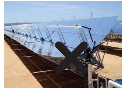
Concentrated solar power
