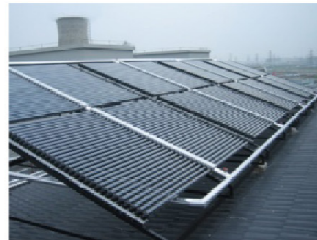
Evacuated tube collectors
