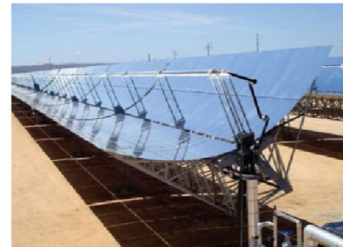
Concentrated solar power
