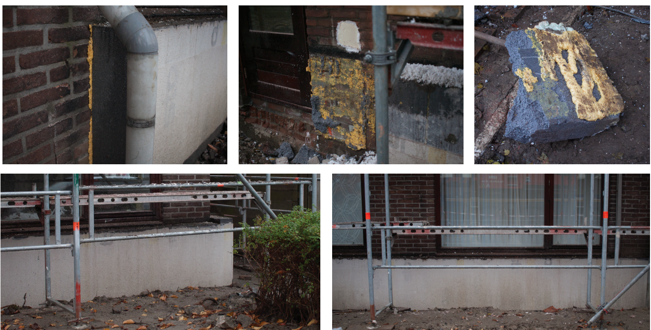
Fig. 42: Photos visit building site Vlaardingen (18-11-2018); placement and removal of EPS insulation board, (source: own photo)
