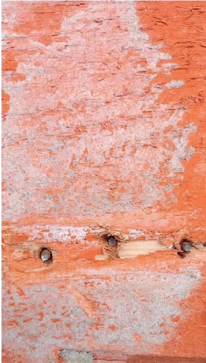
RUSTY SCREWS STUCK INSIDE THE FIBERS
