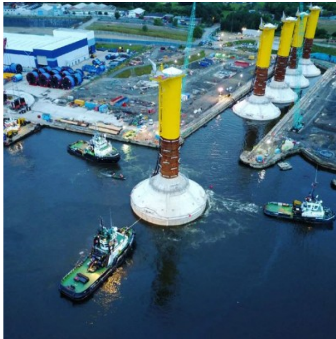
Figure 4.17: Float out of gravity based foundation for float and submerge method used at Blyth offshore wind farm [57]
