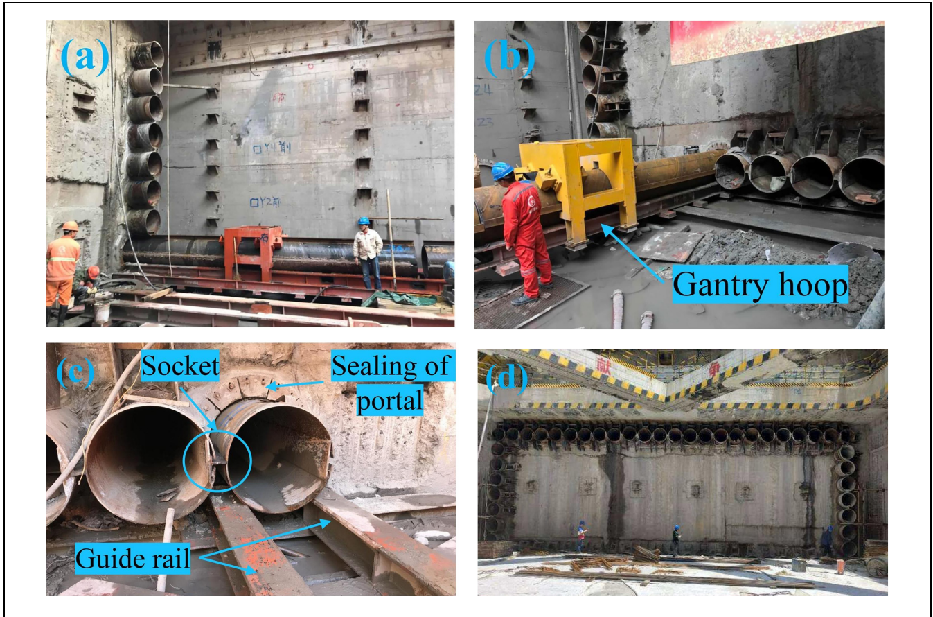
Figure 28. Pipe umbrella installation in the field (25): (a) jacking of the pipes on the right side, (b) gantry hoop for pipe end restraining, (c) jacking of the pipes on the downside, and (d) completion of the whole pipe umbrella.
