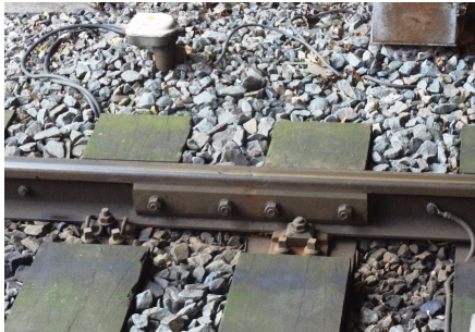
(a) An insulated joint at Utrecht Centraal Station.
