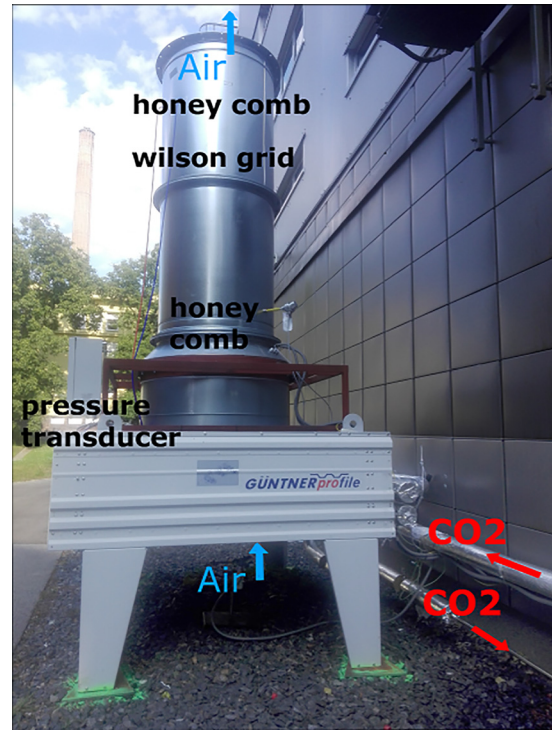
Fig. 6 The sink HX with measurements
