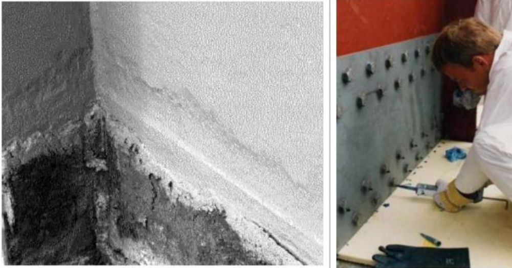
Figure 23.2 Corrosion of steel structure and subsequent repair with injection bolts [5].
