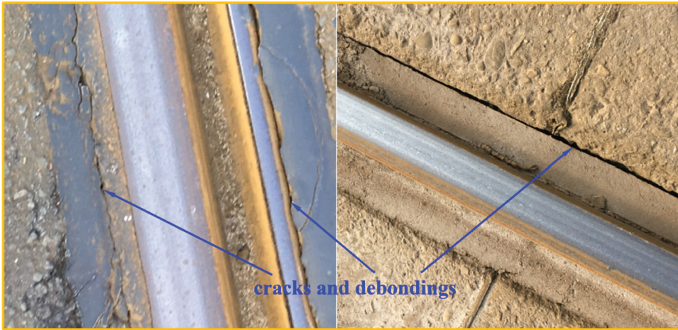
Figure 6. Cracks and debondings observed at operating lines.
