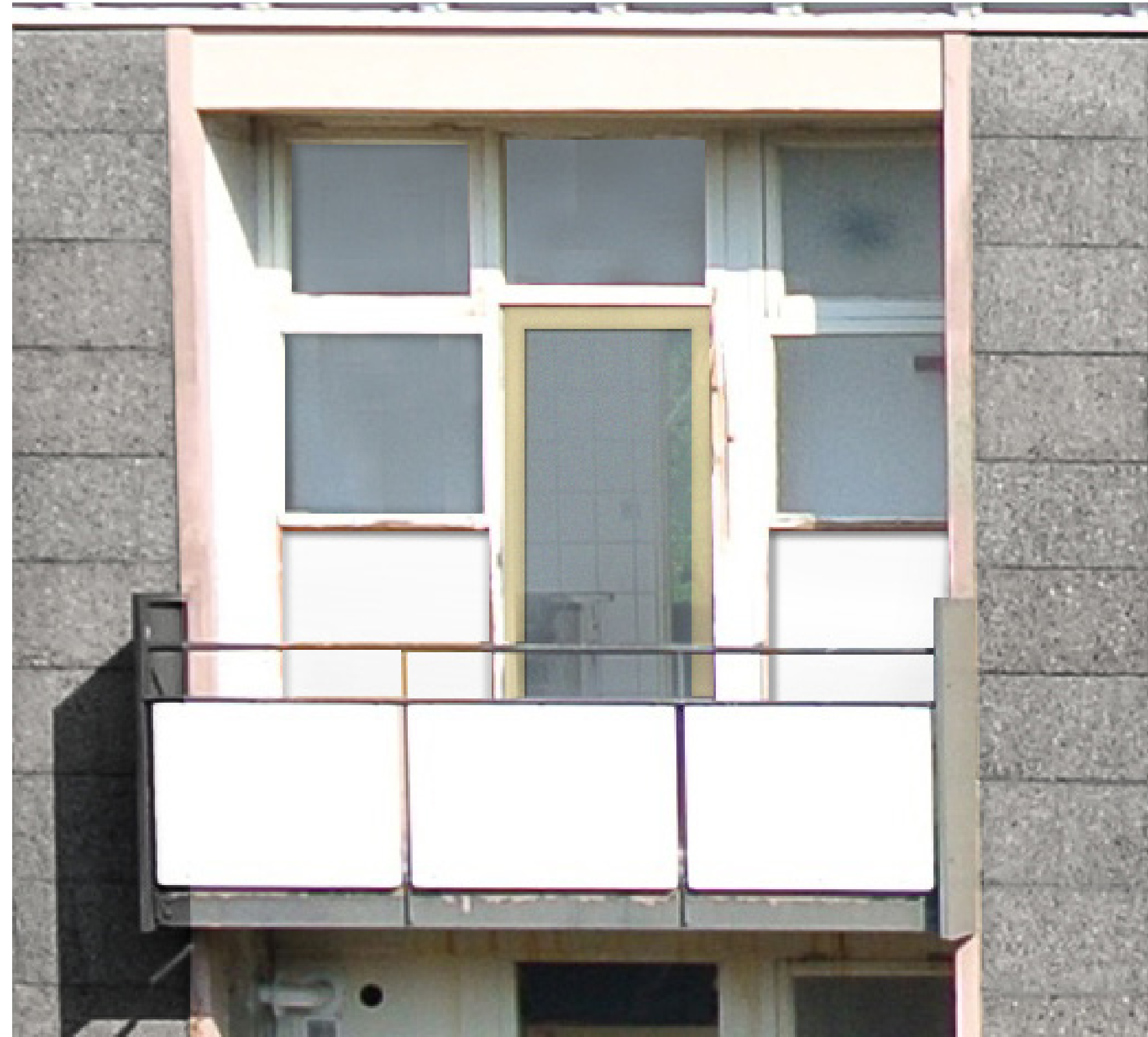
OLD BALCONY (2650 X 1100) Not functional, too small, rotten
