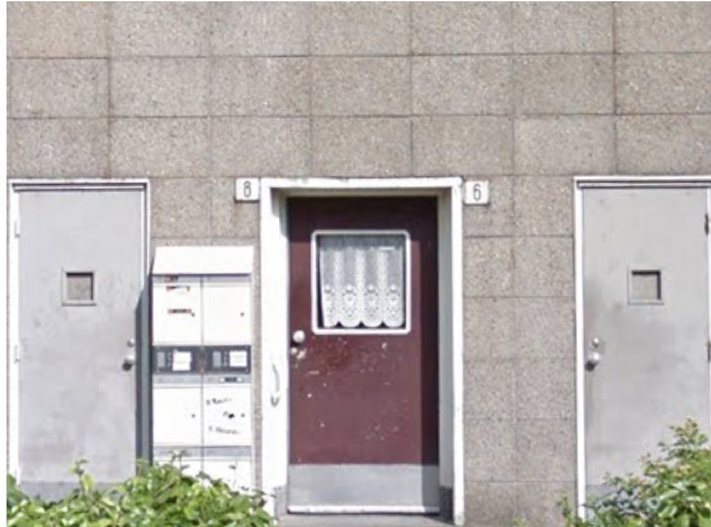
EXISTING ENTRANCE Entrance is not clearly marked
