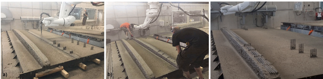
Fig. 10. (a) Add-on Printing of concrete ribs with varying cross-section heights (b) Application of the longitudinal reinforcement bars (c) Application of the concrete cover onto the reinforcement [29].
