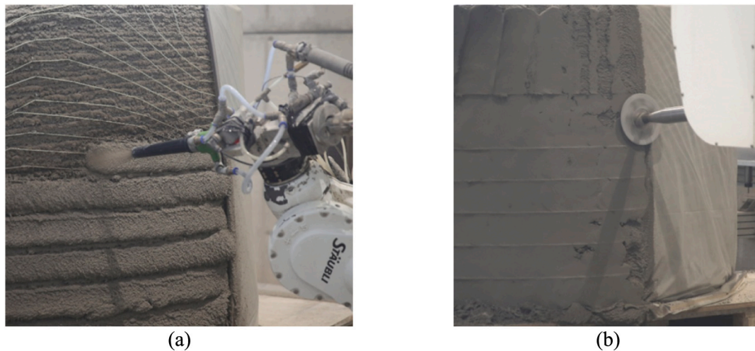
Fig. 24. Printing vertically onto a horizontally printed core: a) embedding the robotically fabricated fibre reinforcement; b) robotically trowelling the fresh concrete in a subsequent formative process, [101].
