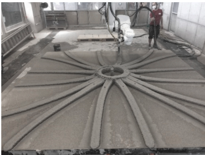
Fig. 5. Add-on Printing of force-flow-optimised concrete ribs of a point-supported slab [27,29]. The concrete ribs have varying cross-section heights according to the course of the bending moment (Technical University of Braunschweig, 2019).
