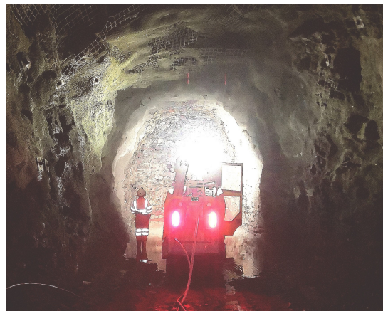
Figure 2.13: K1060 access support method of split sets and rock bolts with mesh as well as 75 mm of shotcrete. Field of view is 5 m.
