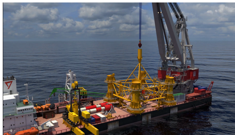
Figure 2.4: Current PIF on deck of with ILT in slings of the crane
