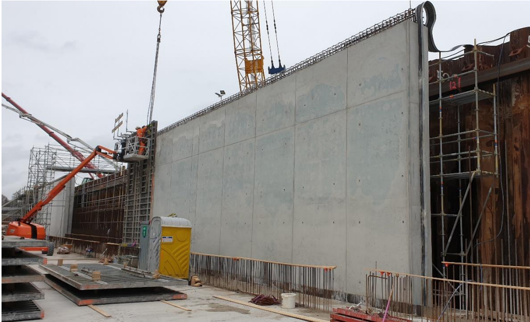
figure 121 Demoulding of the Southern wall of segment 12 of the dive-under during inspection number 1
