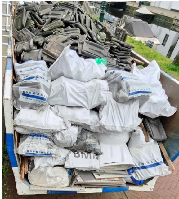
Figure 4.1: 10 m 3 skip found in Leiden containing mostly roof tiles and other roof-waste.
