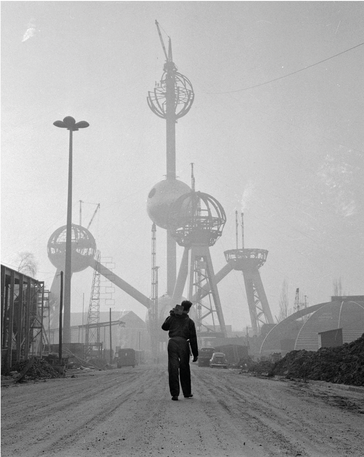
Construction of the Atomium - a symbol of faith in science and the future. Built for the Expo'58 in Brussels.
