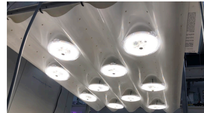
Picture 93,94,95,96,97: Lamps attached to roof, Interface for control Pixel lights, Purple Pixels, Bleu Pixels, Raspberry Pi controlling the Pixels.
