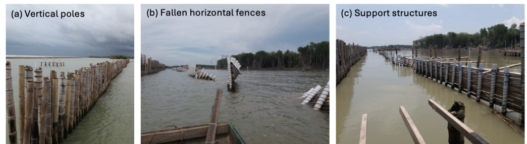
Figure 10. Photographs documenting the repair process of the damaged temporary permeable structure during early 2022: (a) the first row, consisting of vertical bamboo poles embedded in the muddy seabed, remained stable throughout the storm season; (b) the second row, originally constructed with horizontal bamboo poles supported by vertical poles, collapsed in January 2022 due to insufficient stability to withstand wave loads. The damaged sections had a length of 12 m (~30% of the back row) of T3 and 35 m (entire back row) of T4; (c) the structure was repaired between March and April 2022, with the collapsed components lifted and additional support structures added to enhance stability.
